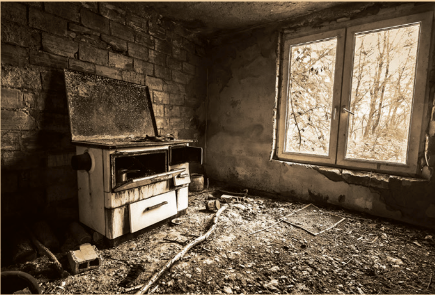
Burned Roma House in Trubari Settlement, Srebrenica Municipality
